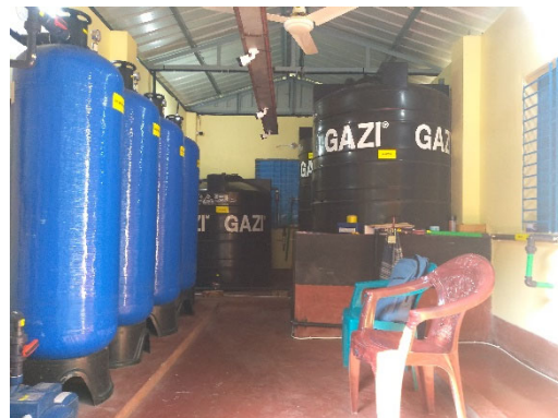
Water treatment facility
